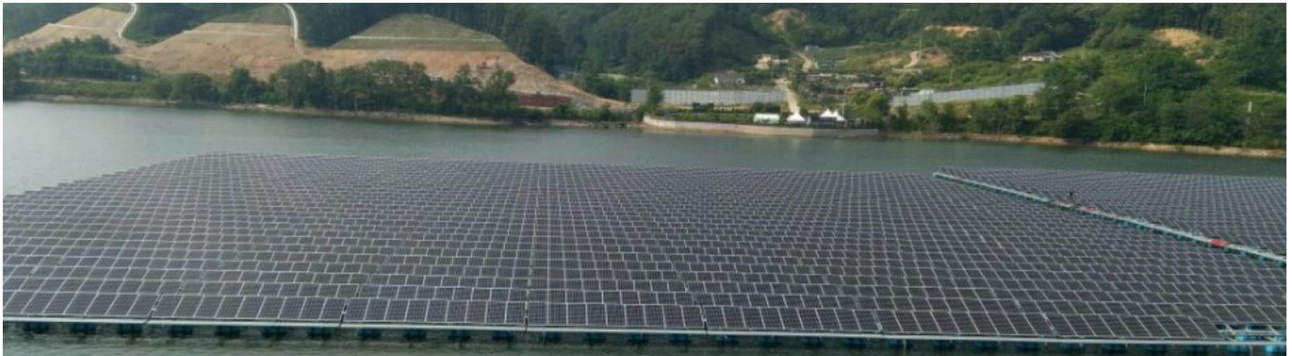
Sosoo plant (Lake) 2MW
